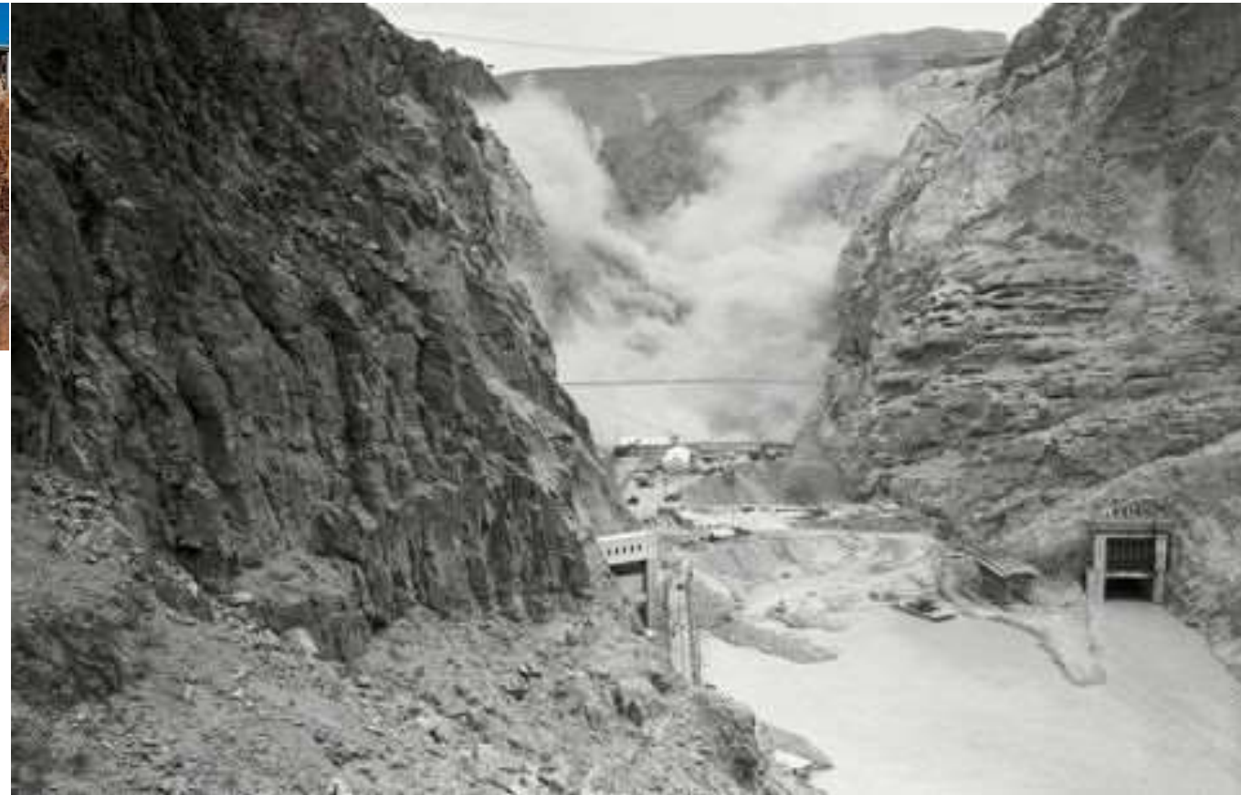
A 4-Ton dynamite blast during construction of the Hoover Dam on May 12, 1933, in Nevada. Bettmann/Getty Images
